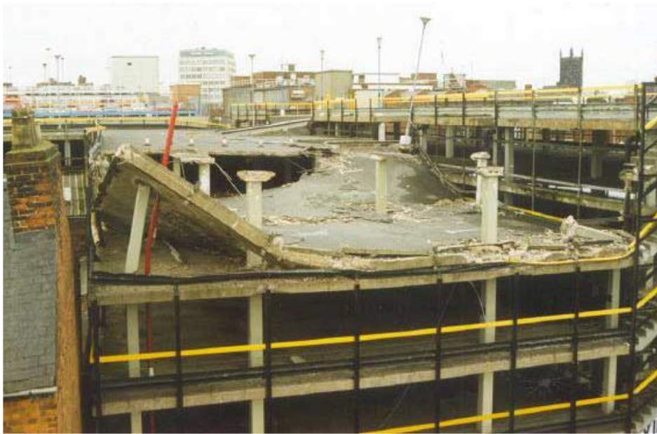
Figure 6. Top story collapse at Pipers Row Car Park, UK. (Wood, 1997)
